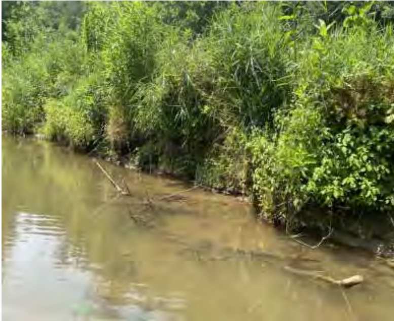
Erosion Area 13: “Moderate”
