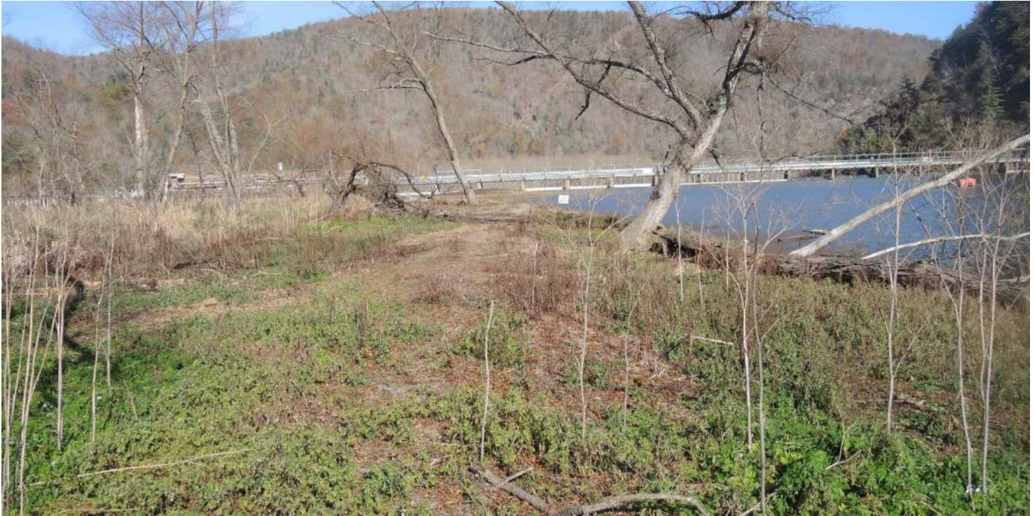
Photo 3-11: Section of trail near the portage take-out is grown over with vegetation and needs to be resurfaced to provide sufficient walking surface and to clarify trail route.
