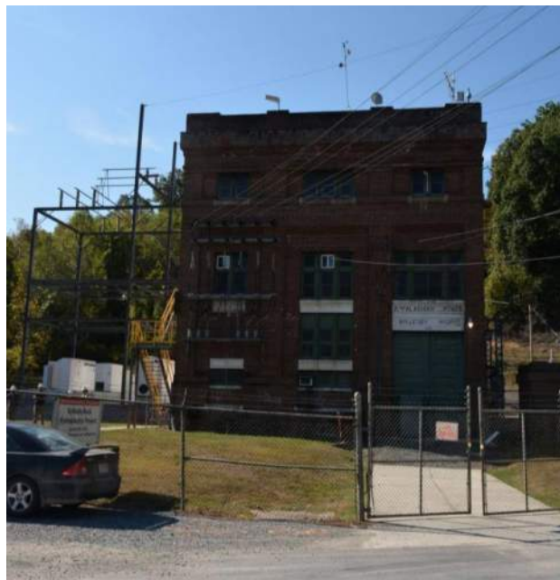
Figure 1. Byllesby control house, exterior switchyard (at right), and battery system (at left).
