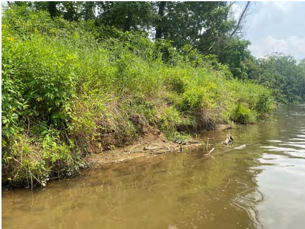
Erosion Area 4; Category “High”
