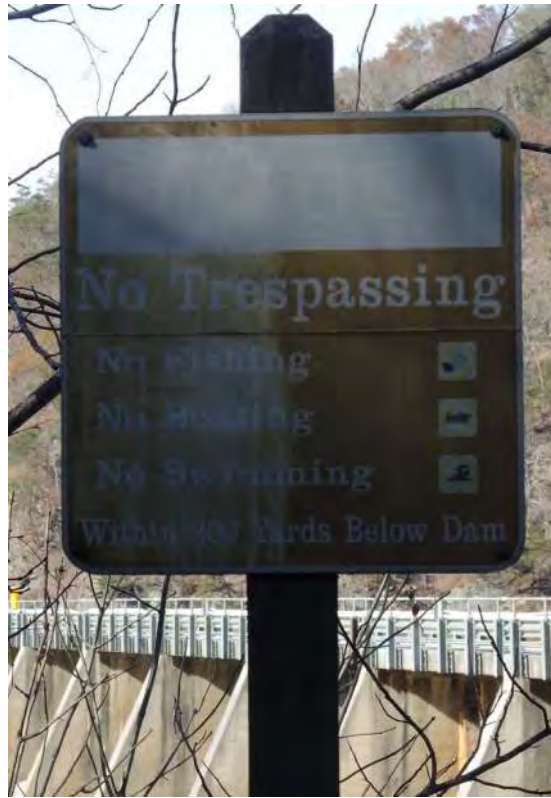
Photo 6-6: Faded regulations sign
