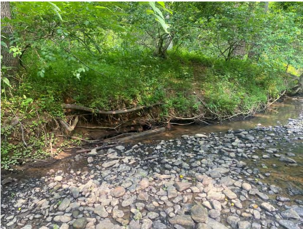
Erosion Area 2; Category “High”
