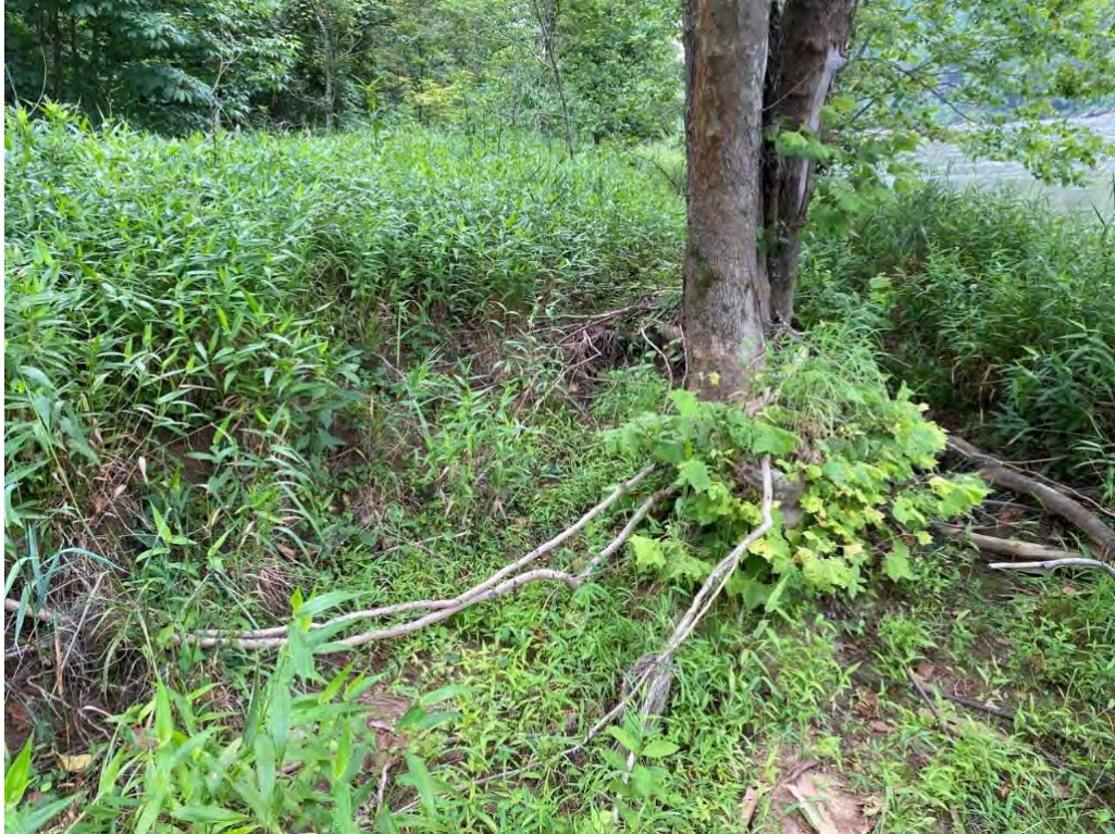
Erosion Area 15; Category “Low”
