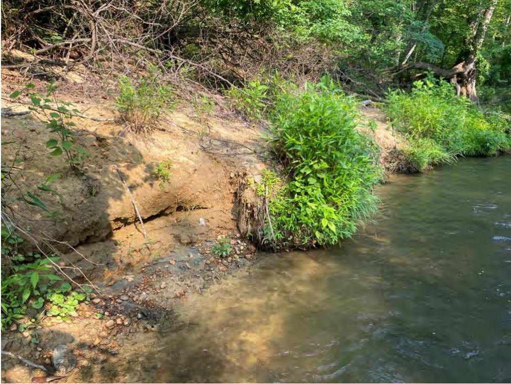
Erosion Area 1; Category “High”
