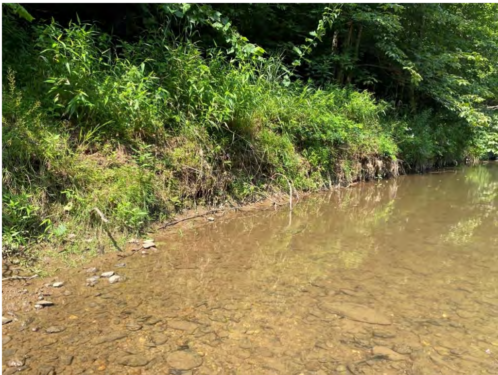
Erosion Area 10; Category “Moderate”
