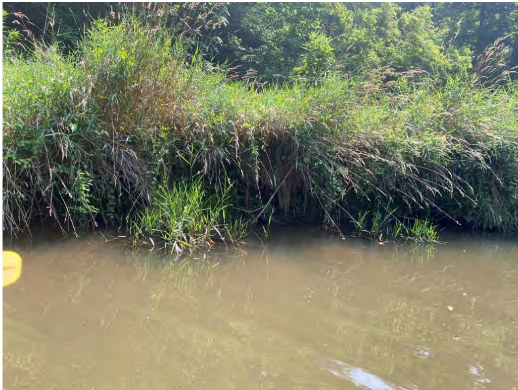
Erosion Area 12; Category “Moderate”
