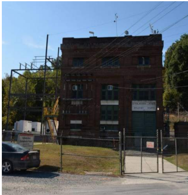
Figure 1. Byllesby control house, exterior switchyard (at right), and battery system (at left).
