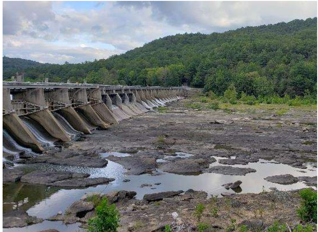
Buck Bypass Reach 9.9.2020 Leakage Flow
